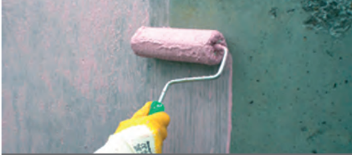
High adhesion between concrete and cement render
